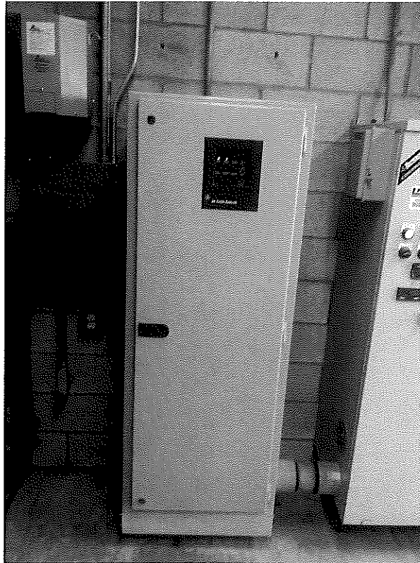
The 3 conduits connects to the 3 control panels. The grey is the switching for the generator, the off-white is the control panel for the electric water well pump, and not pictured is the Edison panel.
