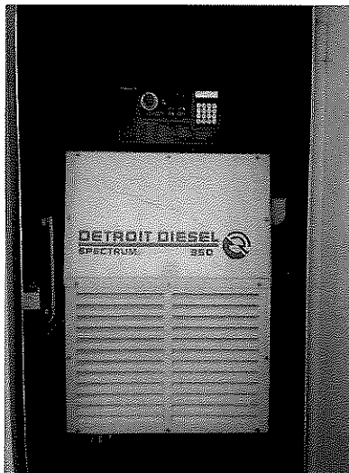
The above is the photo of the actual generator inside the exterior housing.
